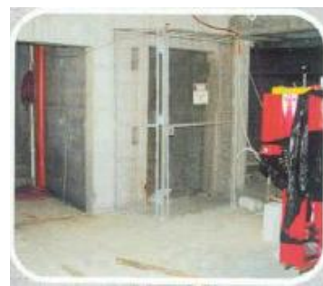
Puțuri de lift
